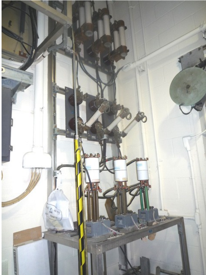
14.4kV 3-phase isolators
