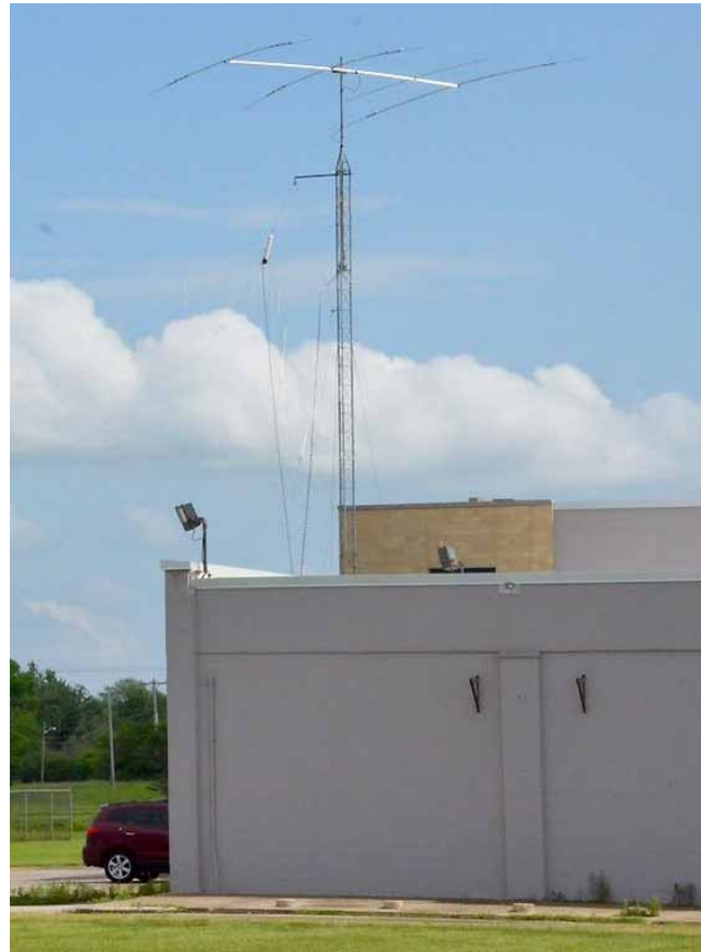
HF Yagi & wire antennas on tower
